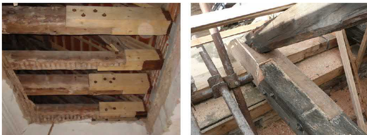
Figure 8. The use of metal fasteners in timber end replacements in Buštehrad Castle, Czech Republic [22, p. 68].
