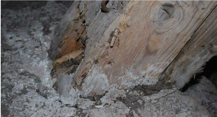
Figure 3. Rotten rafter S18 penetrating to the masonry wall.
