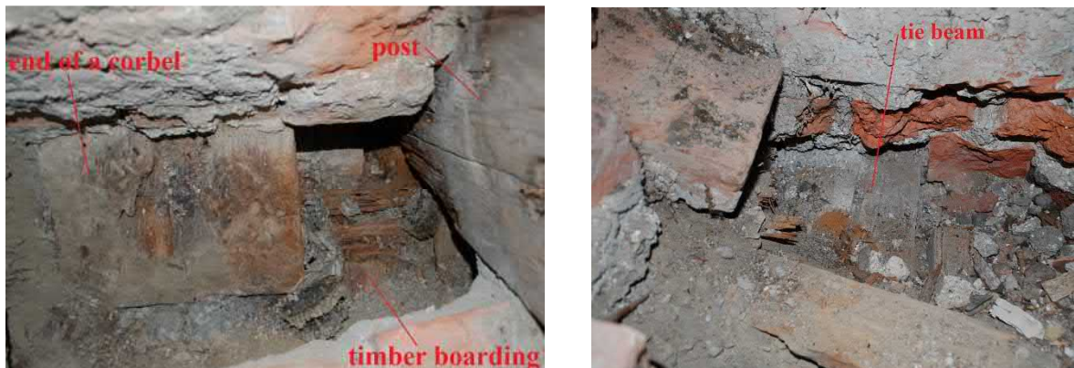
Figure 32. Structural openings that have been made in the attic. The left one is in the southeast and the right in the southwest side of the roof.
