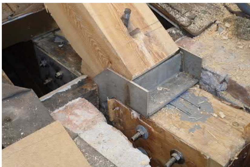
Figure 49. Repair of a tie beam end in 2010 in the catholic church located in Helsinki. The rotten end of the tie beam supported by masonry wall was replaced with a new timber piece and the connection between members was implemented with steel plates and bolts. Birch bark was installed to the surfaces of timber member, and air gaps surrounding the member were left to improve the durability of the structure. [55]
