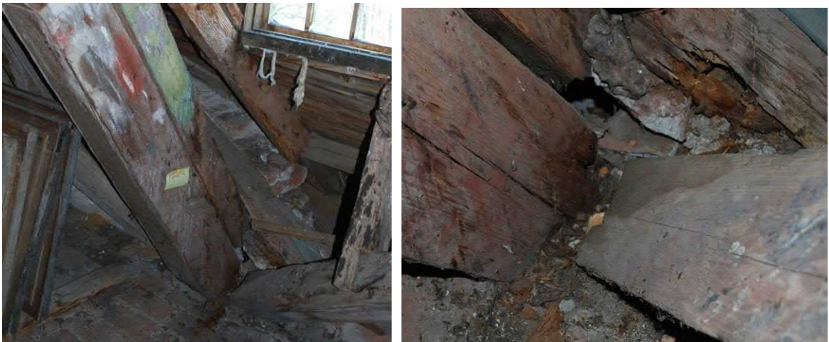
Figure 5. Left: post of the leaning trestle (PIIIII), rafter (S41), cross bracing and the diagonal timber member that reaches to the top of the gable. Right: showing the stage of decay more detailed. Rafter has lost its entire cross section.
