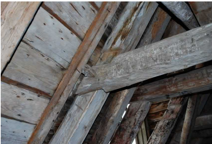
Figure 34. Connection that has lost its structural capacity. Original markings can be seen on the side of the rafter. Also, one collar beam is entirely missing from its place which can be due to obstacles in between the rafter pairs. See detail C in Figure 18.
