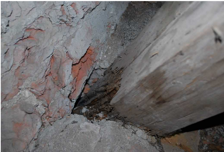
Figure 35. Rotten rafter S29 penetrating to the masonry wall.
