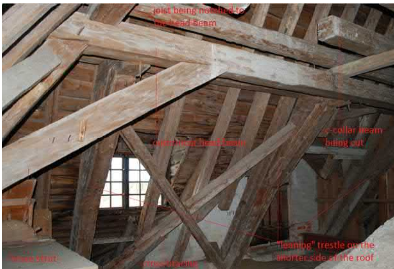
Figure 21. The outermost leaning trestle which spans across between the long external walls is supporting the leaning trestles on the shorter side. Cross bracings can be seen between leaning trestles. The cross bracings are missing where the gables are located. One of the collar beams have been cut due to previous lead through.
