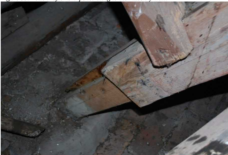
Figure 36. Previous repair intervention on the end of the rafter S43.
