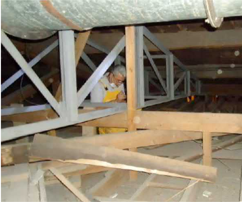
Figure 15. Additional steel roof trusses are installed to increase the load-bearing capacity of the timber roof structures [49, p. 5].
